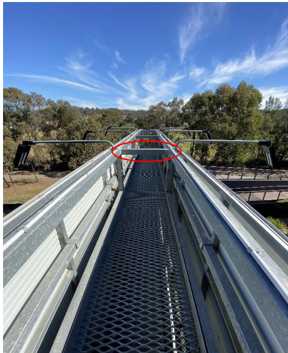
Photo 15 – Trip hazards to top catwalk (circled).
